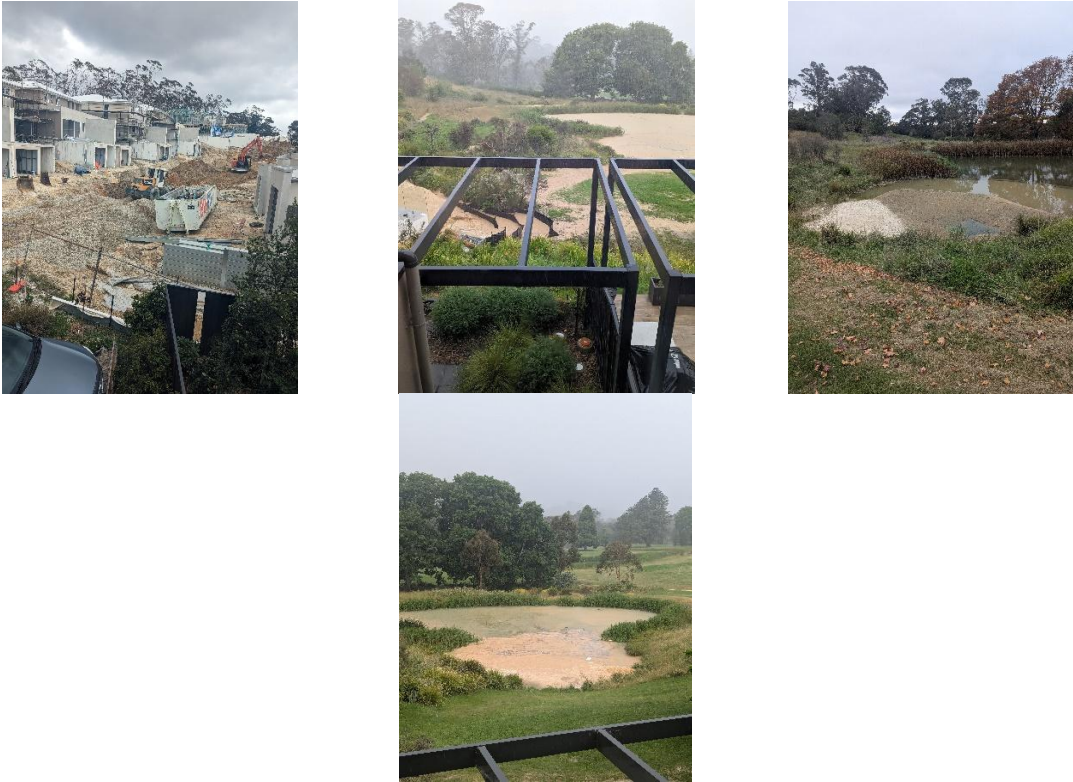
Figure 3.2: From left to right; the adjoining Escarpments development, stormwater breaching sediment fencing; resulting sedimentation and pollution of the adjoining watercourse. Source: Jennifer Buick.
